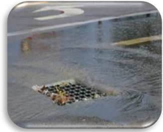
Photo: Road stormwater collection
